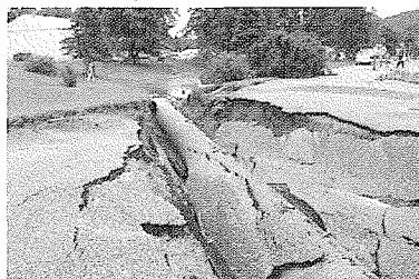
Damage to a road caused by flood water. The road collapsed around a drainage pipe that ran under the road.
