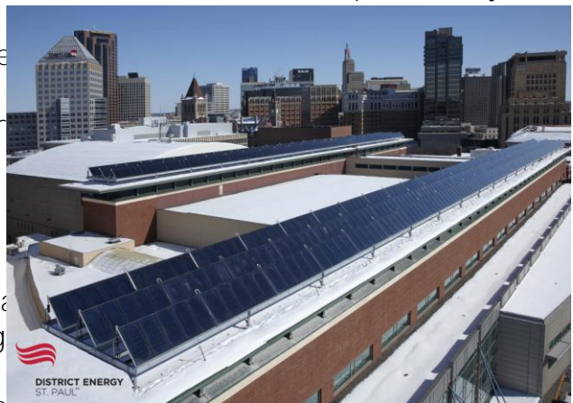
Photo credit: District Energy St. Paul
