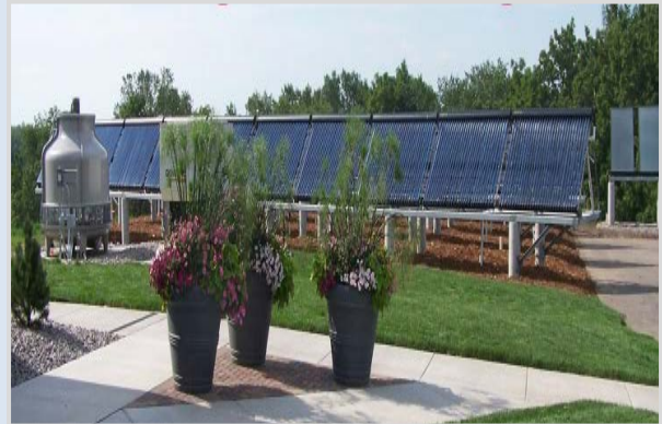
Figure 6. Evacuated tube array outside of WCROC
