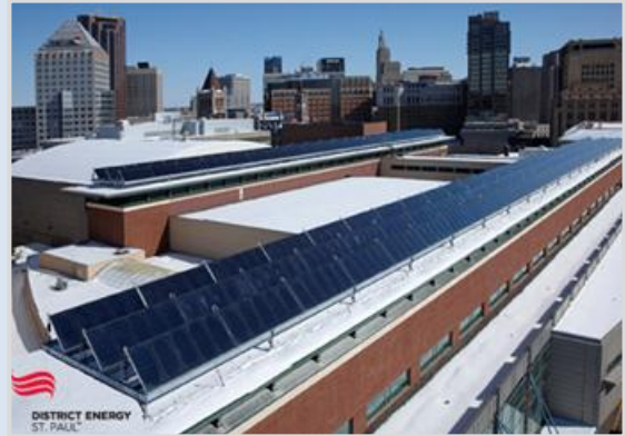
Figure 7. The District Energy St. Paul is the largest solar project in the state
